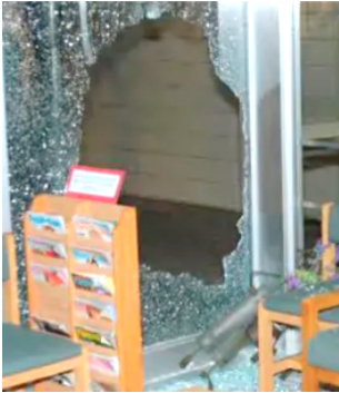
(L) The broken window
